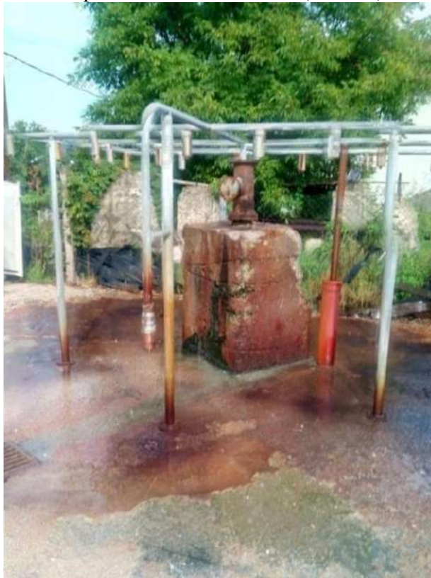
Figure 3. View of the mouth of the borehole SI-1 in Slavinovici, with the construction of the choke manifold (showers) (Photo: Nuhanovic, S; Barusic, B., 2020.)
