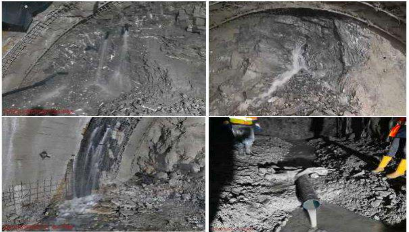
Figure 2. The emergence of underground water in the Zenica tunnel
