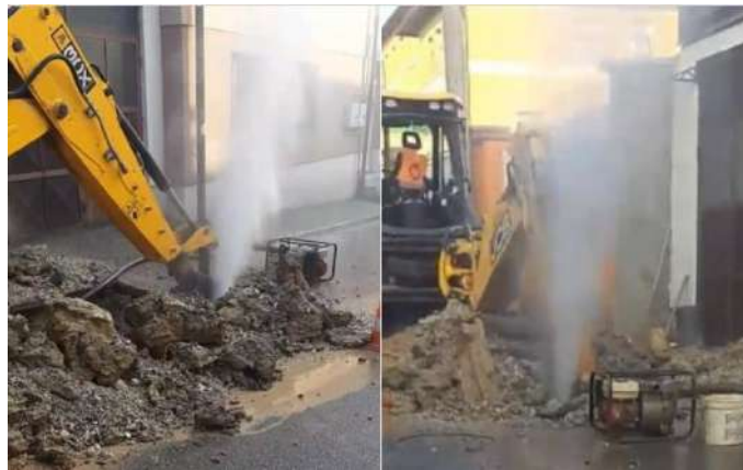
Figure 5. Damaged gas pipe (Source: https://www.faktor.ba )
