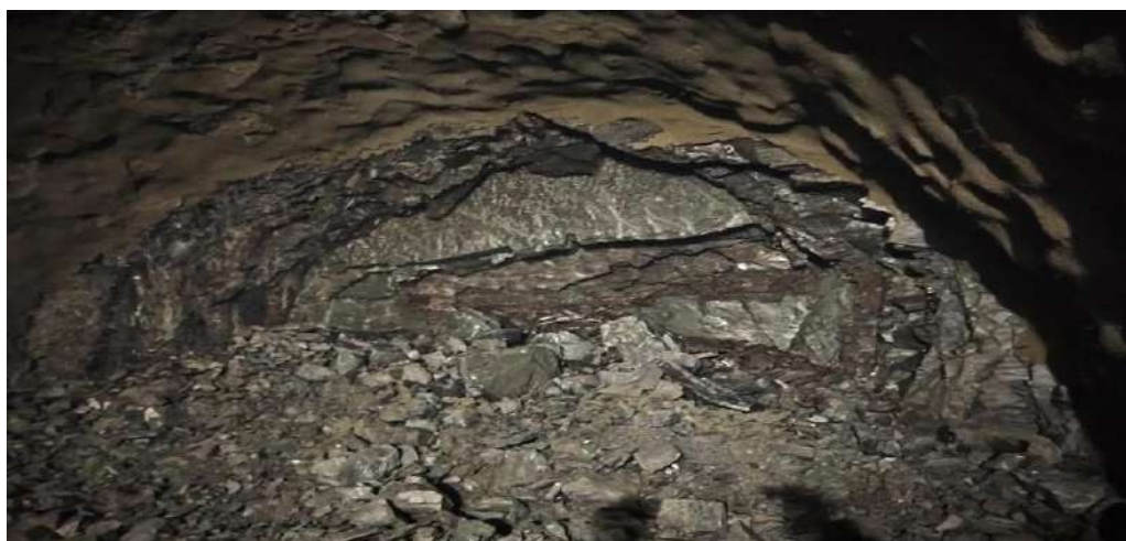
Figure 5. Fallout of rock blocks in the Zenica tunnel
