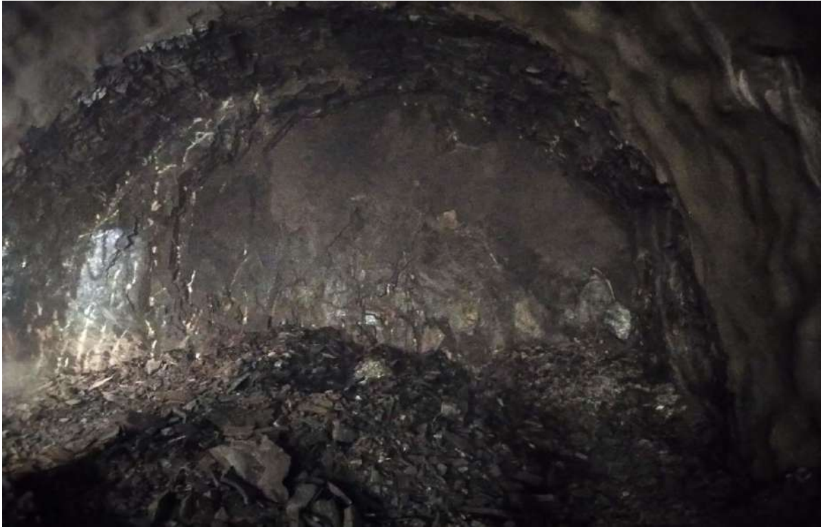
Figure 10. LTT face cross section at chainage 1+524.088 after blasting and treatment of the cross section
