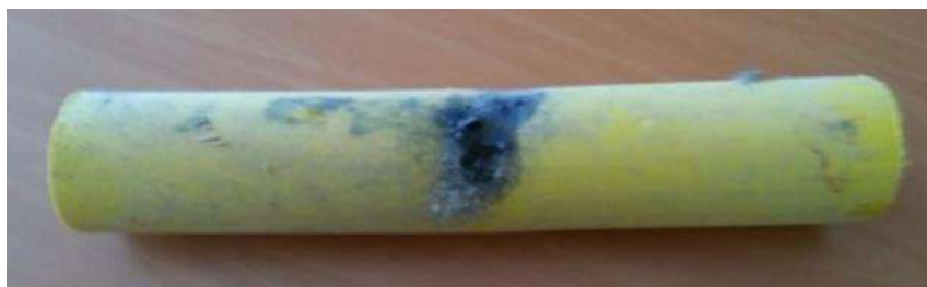
Figure 4. Damaged gas network pipe
