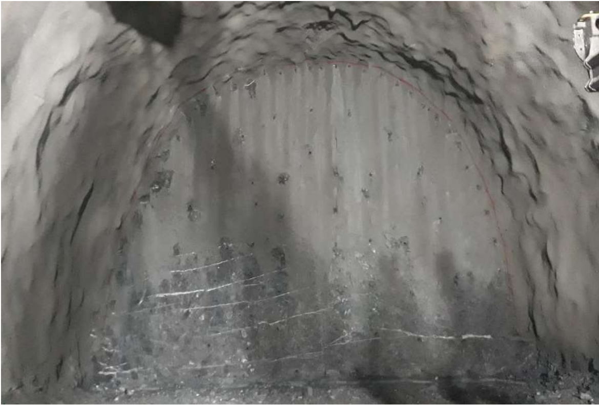
Figure 9. LTT face cross section at chainage 1+522.08 after completion of drilling of all blast holes according to the defined scheme
