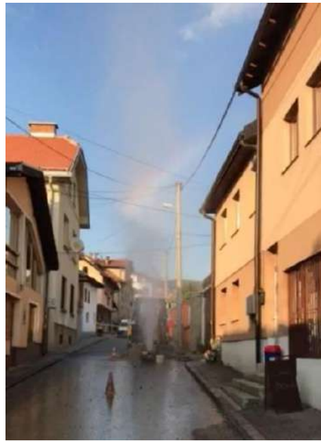
Picture 6. Damaged gas network pipe in the settlement of Bjelave
