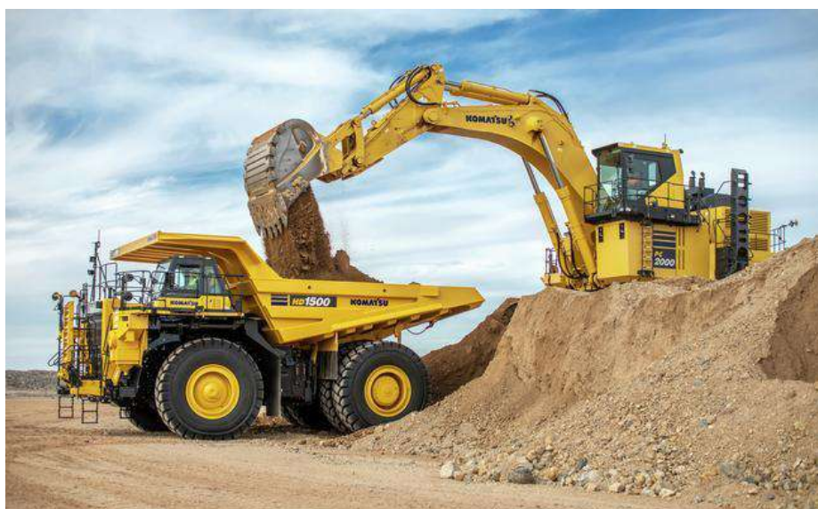
Figure 3. Loading material with a hydraulic excavator with an inverted bucket into a truck - bottom digging
