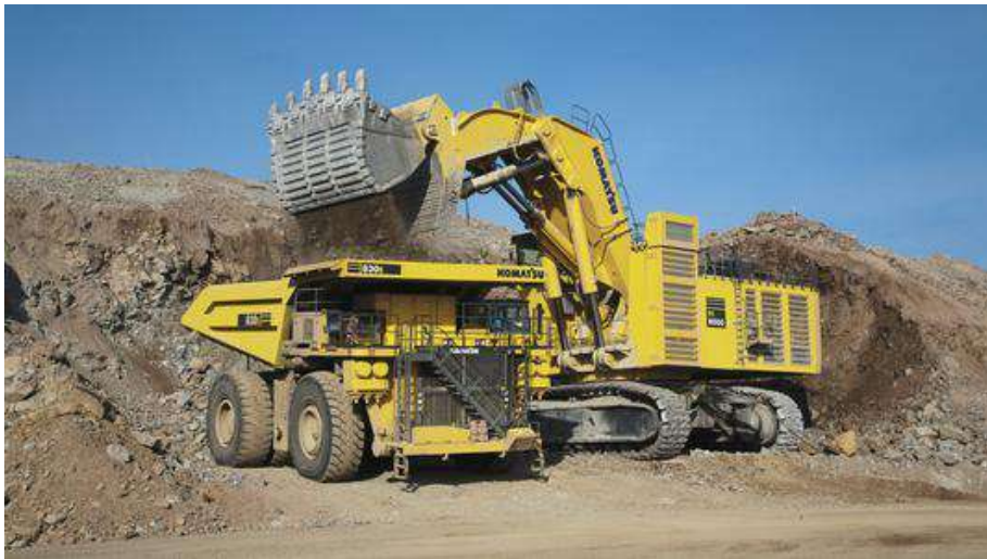
Figure 2. Loading material into a truck with a hydraulic excavator with a folding bucket
