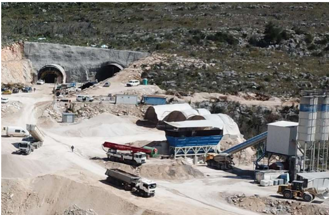
Figure 4. Layout of the installed concrete plant for concrete production [6]
